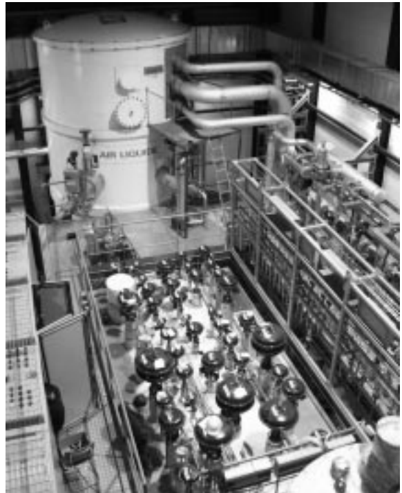
Figure 5: Coldbox of first 18 kW @ 4.5 K helium refrigerator
